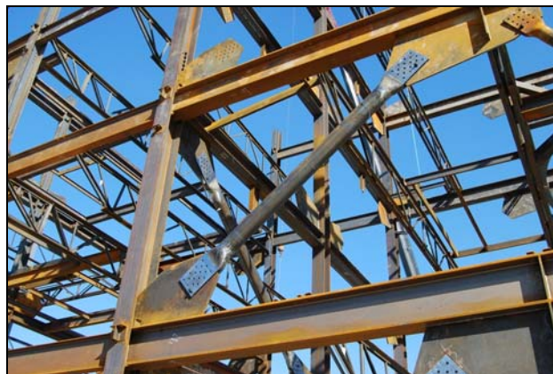
Caption: Brace equipped with Cast ConneX™ High-Strength Connector installed in frame during initial structural erection phase.
